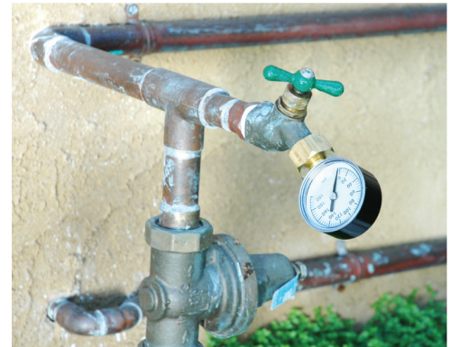
Figure 4 - Water Pressure Gauge
